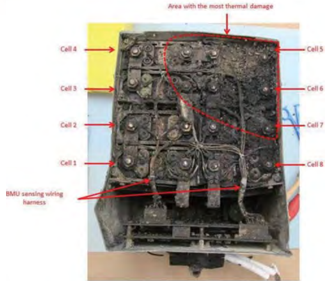
Figure 10. Thermal damage to battery.
